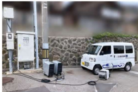
▲ Manhole pump start-up support system for power failures
